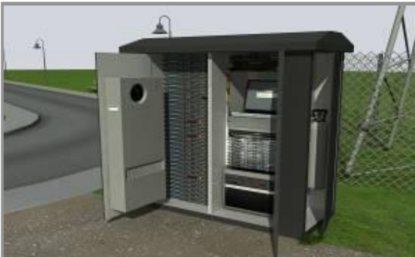
Back up power, e.g. Telecom
